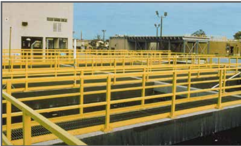
Square tube railing manufactured with Dynaform component products offer long life in the corrosive environment of this wastewater treatment plant.
