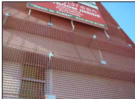
Application: Screening/Sunscreens Product: Fibergrate Molded Grating
